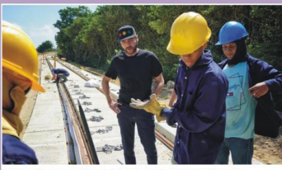
The Bocas de Ceniza train will have 2600 meters of railway track - credit: Mayor's Office of Barranquilla
